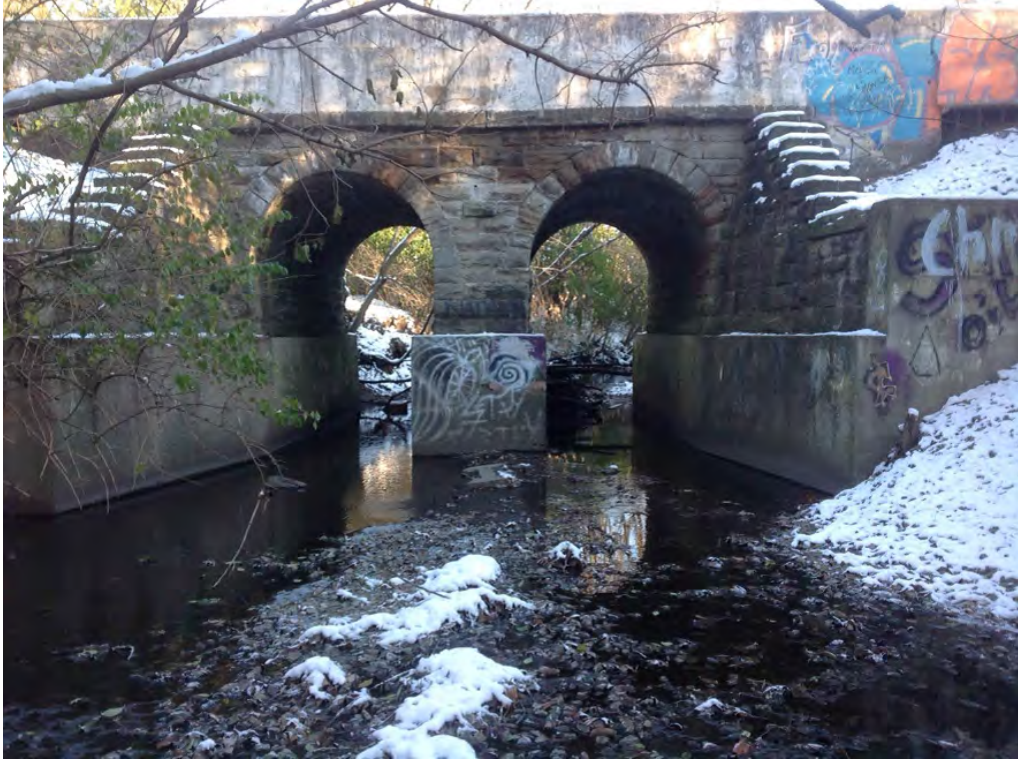
Photo 3: Looking upstream at active railroad bridge between transects 12 and 13. Stream bed consists of sand, gravel and cobbles. Poured concrete floor under bridge arches is completely exposed on RDB side bridge arch.
