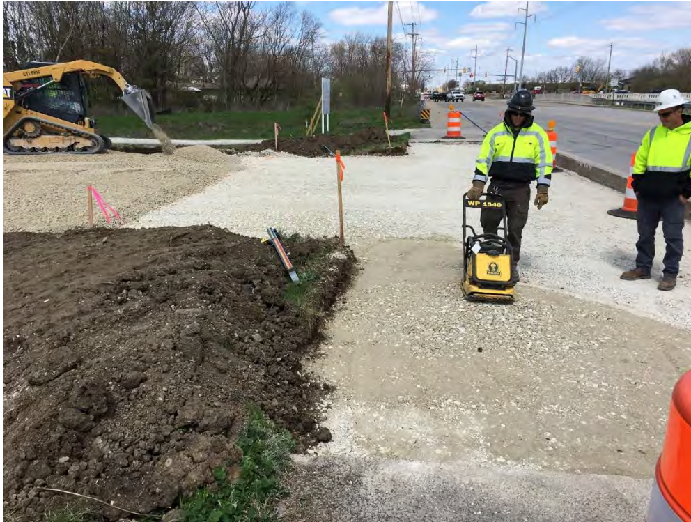
Photograph 2 – EFS preparing subbase grade of pedestrian walking path and drive apron location
