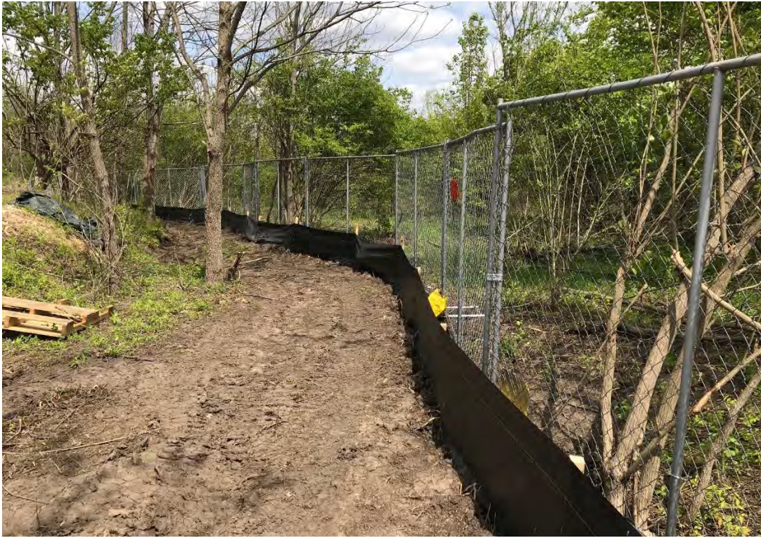
Photograph 2 – Silt fence with branch removed and reattached to stakes .
