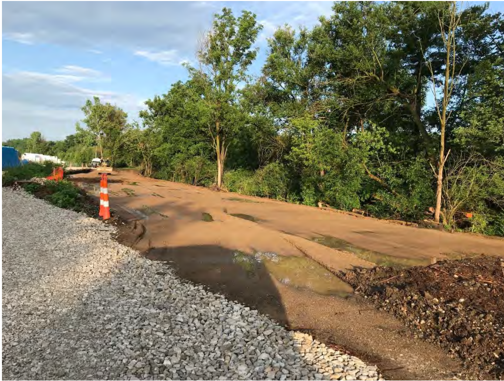
Photograph 2 – Wet backfill from precipitation event.
