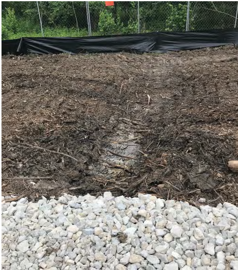
Photograph 2 – Weepers to convey water for the haul road.
