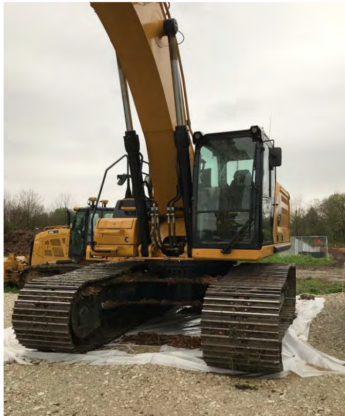
Photograph 1 – Excavator on tarp and gravel pad (no releases to the site/environment observed)
