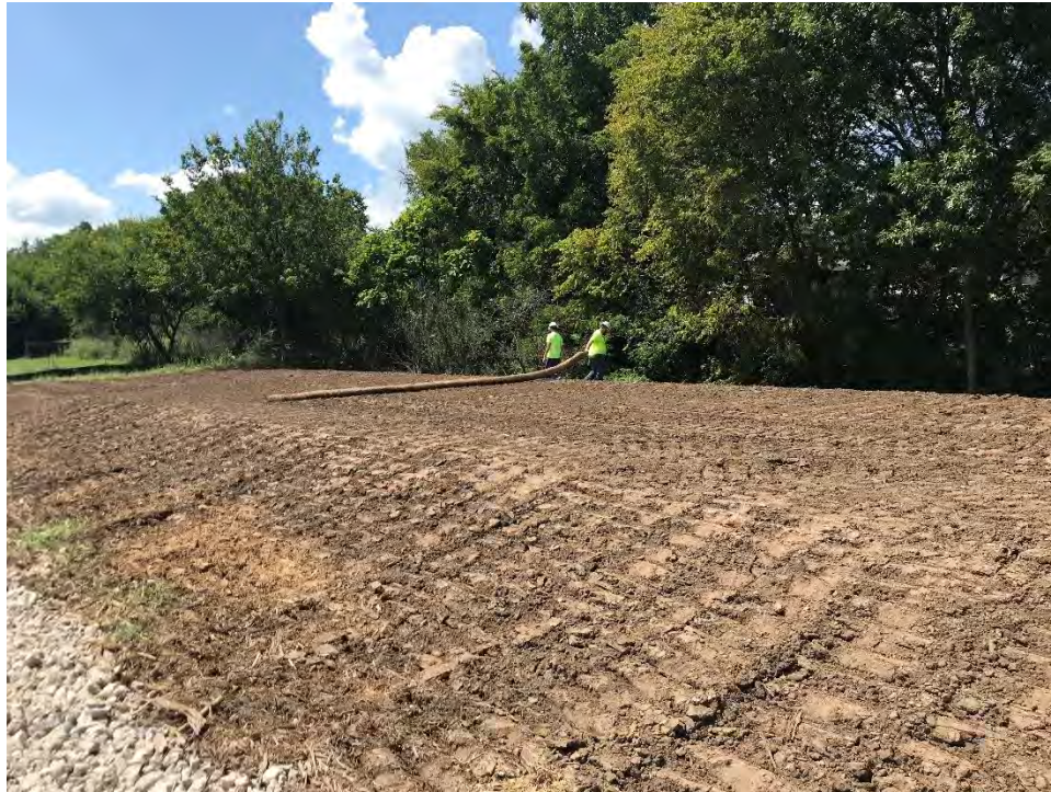
Photograph 2 – EFS installing straw wattles along slope of Elliott Ditch in Area H.
