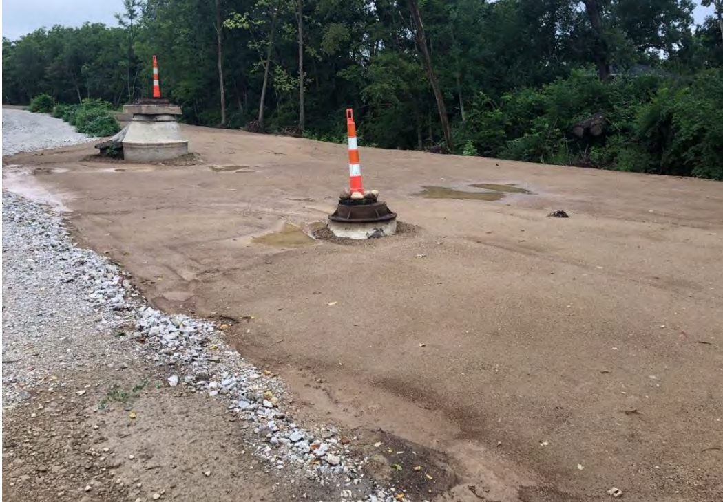
Photograph 1: Standing water in Area B(a) (provided by EFS)
