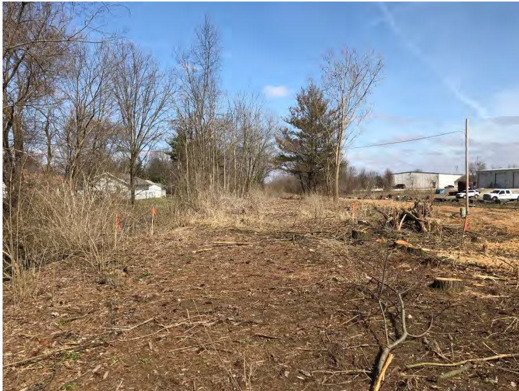
Photograph 1 – Cleared and mulched Area E and no dig area (refer to excavation overview drawing C200)
