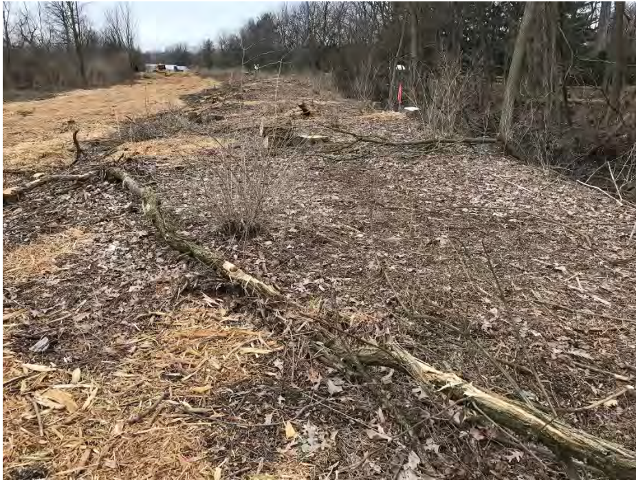
Photograph 2 – Mulch Spread along fence line area and levee where soil was disturbed
