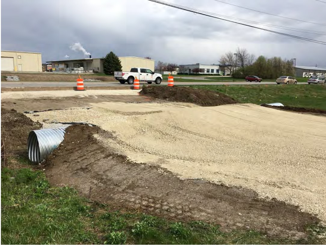
Photograph 4 – Culvert Pipe Install with No. 8 Stone Backfill, Filter Fabric, and No. 53 Stone Overtop
