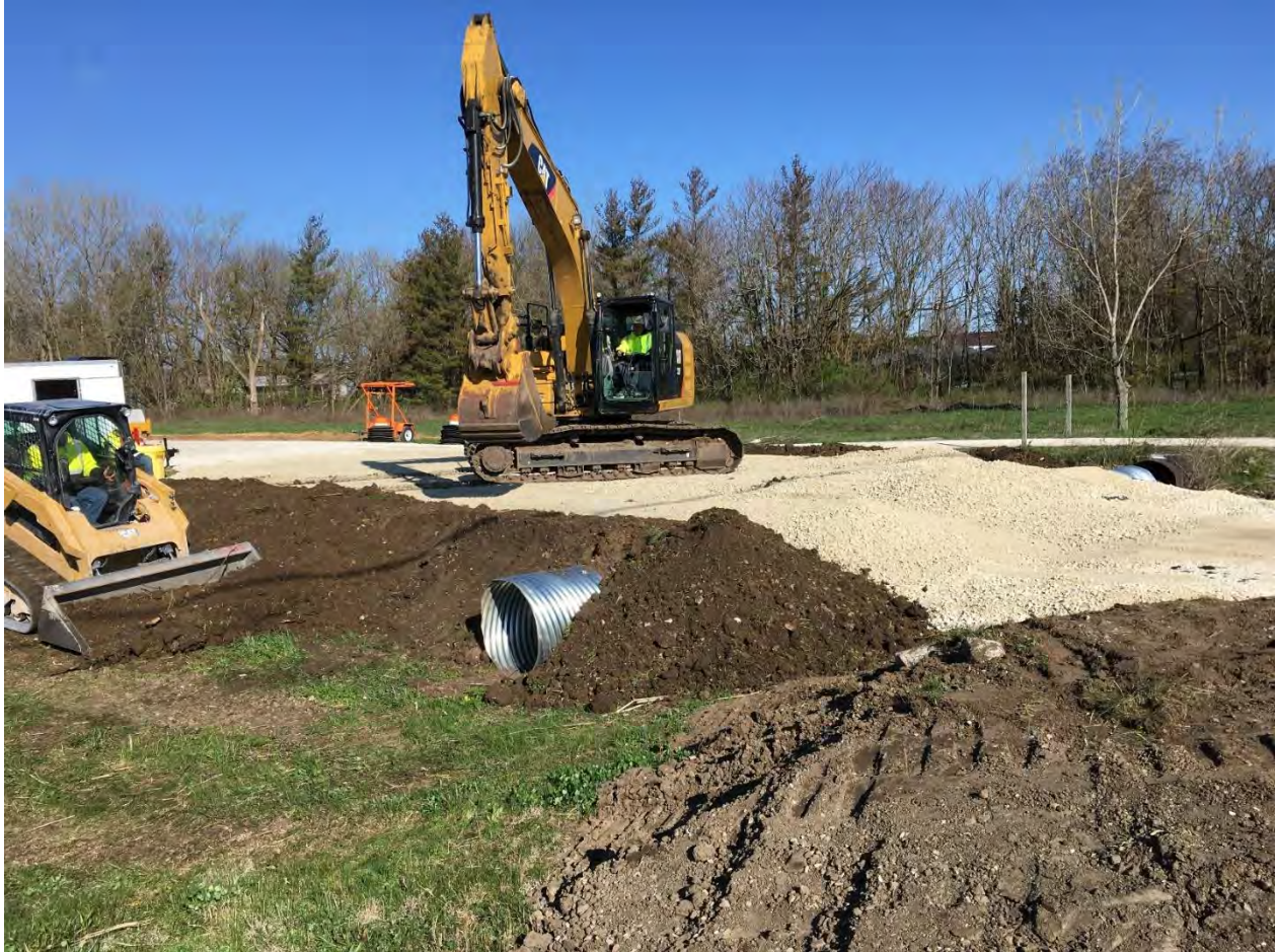
Photograph 1 – EFS continuing fill over culvert with No. 53 stone and grading side slopes with excavated topsoil
