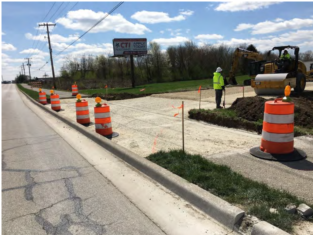
Photograph 3 – EFS finishing subbase grading, ready for Concord Rd. curb removal and concrete forming
