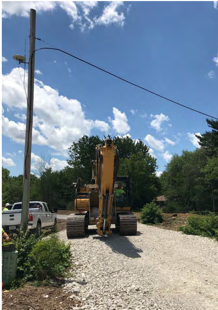
Photograph 3 – Tracking the excavator back to Area C (spotters helping due to overhead telecommunication line).
