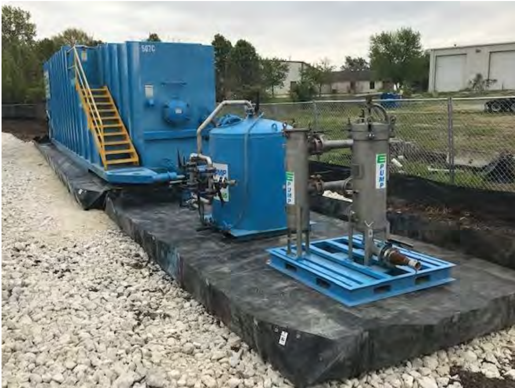
Photograph 2 – Frack tank and water treatment equipment with secondary containment.
