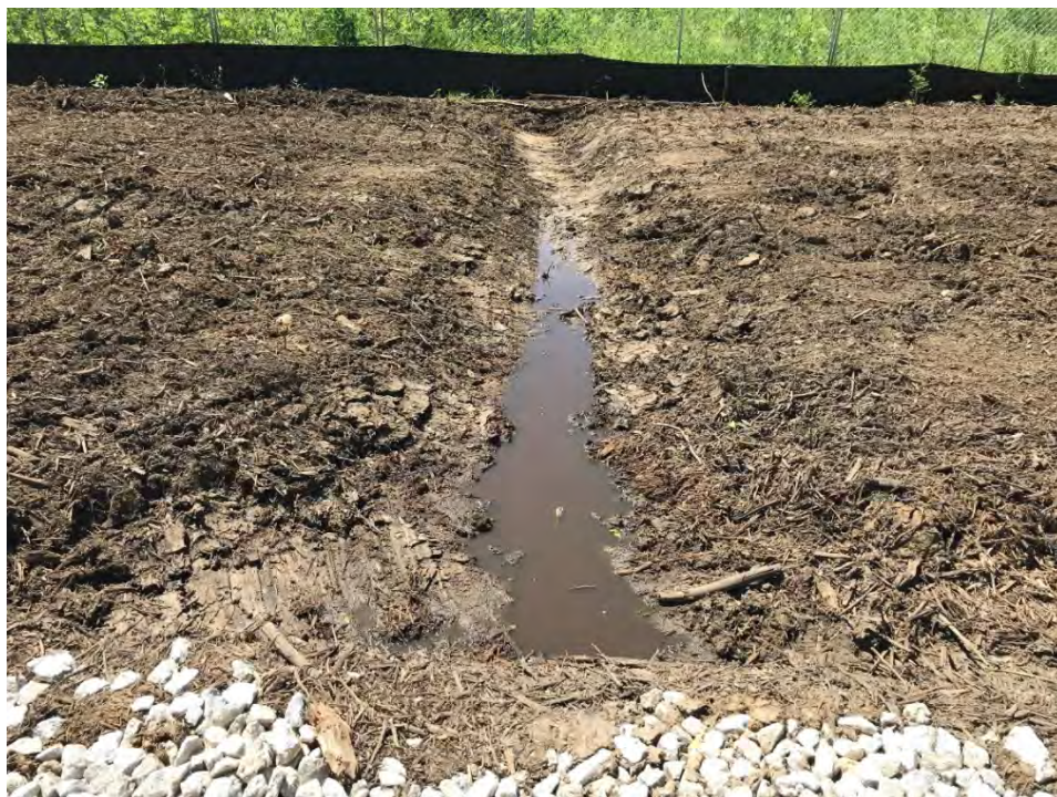
Photograph 2 – Weepers to convey water for the haul road.
