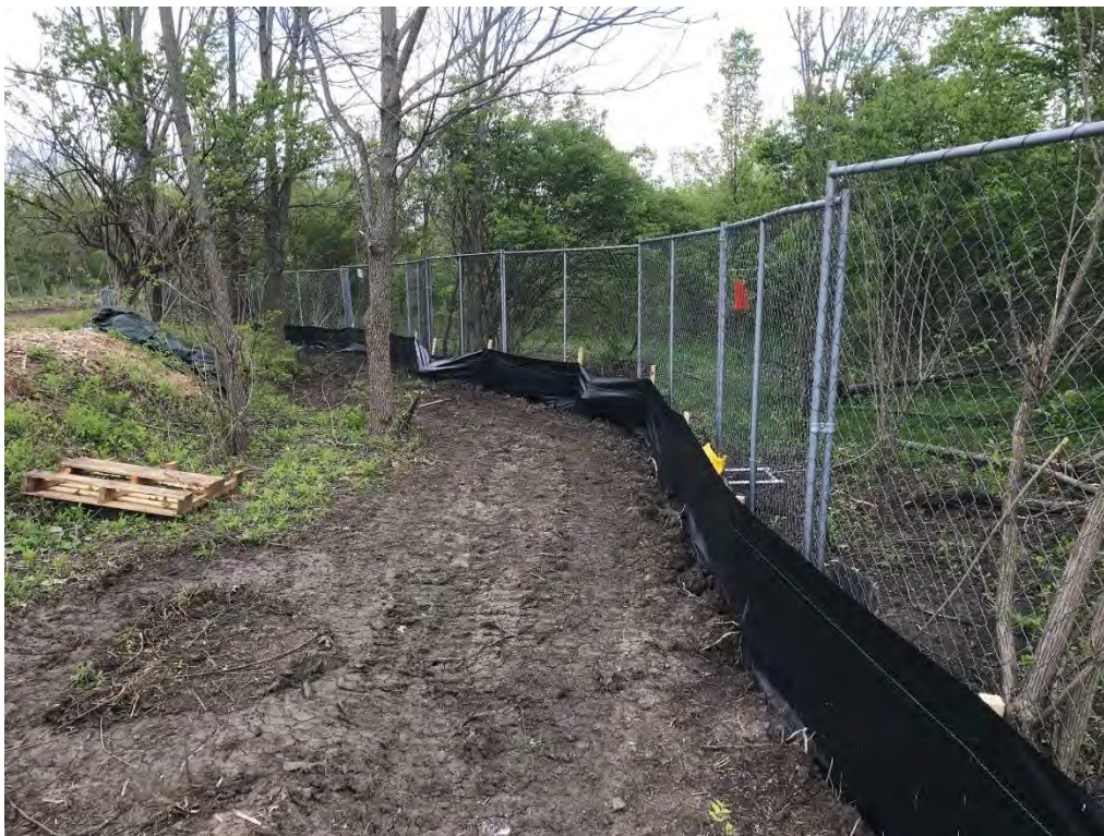
Photograph 1 – Silt fence pulling off stakes due to roots and branches. Repairs completed.
