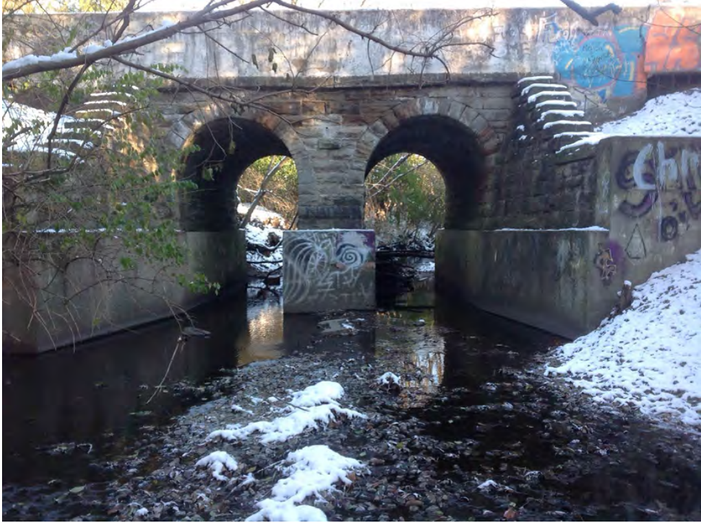
Photo 3: Looking upstream at active railroad bridge between transects 12 and 13. Stream bed consists of sand, gravel and cobbles. Poured concrete floor under bridge arches is completely exposed on RDB side bridge arch.
