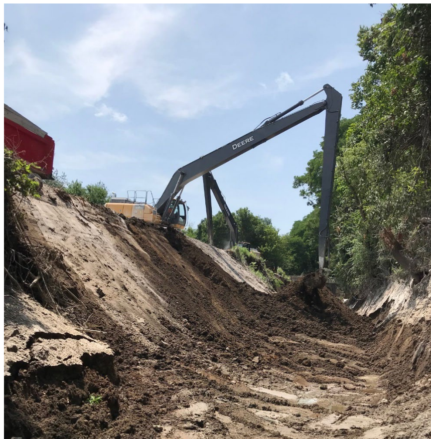
Photograph 2: Over-excavation in Elliott Ditch Reach 1
