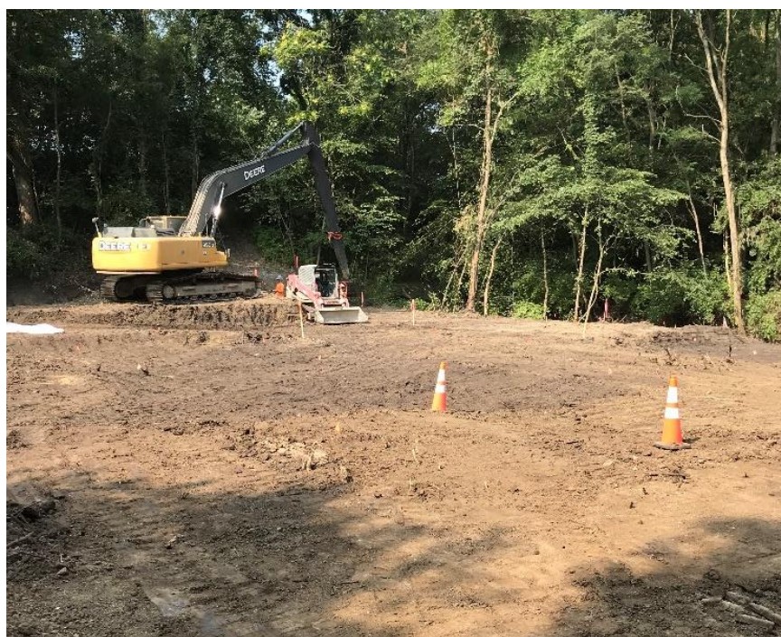
Photograph 1: Soil Excavation Activities in Lower Reach 1, Downstream of the Rail Road Crossing.
