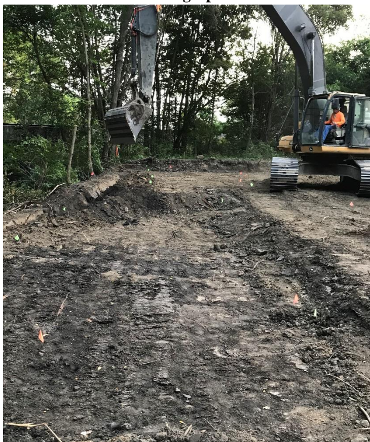
Photograph 1: Over-Excavation Soil Activities in Lower Reach 1, Downstream of the Rail Road Crossing
