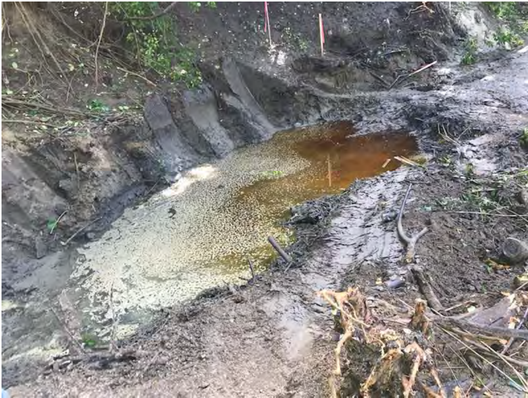
Photo 1: Hydraulic oil on ponded surface water contained in the active excavation footprint
