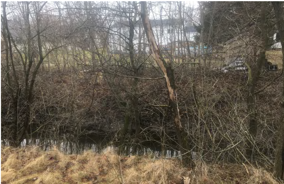
Photo 23: Levee/Elliott Ditch bank conditions, facing west (Location 9)*
