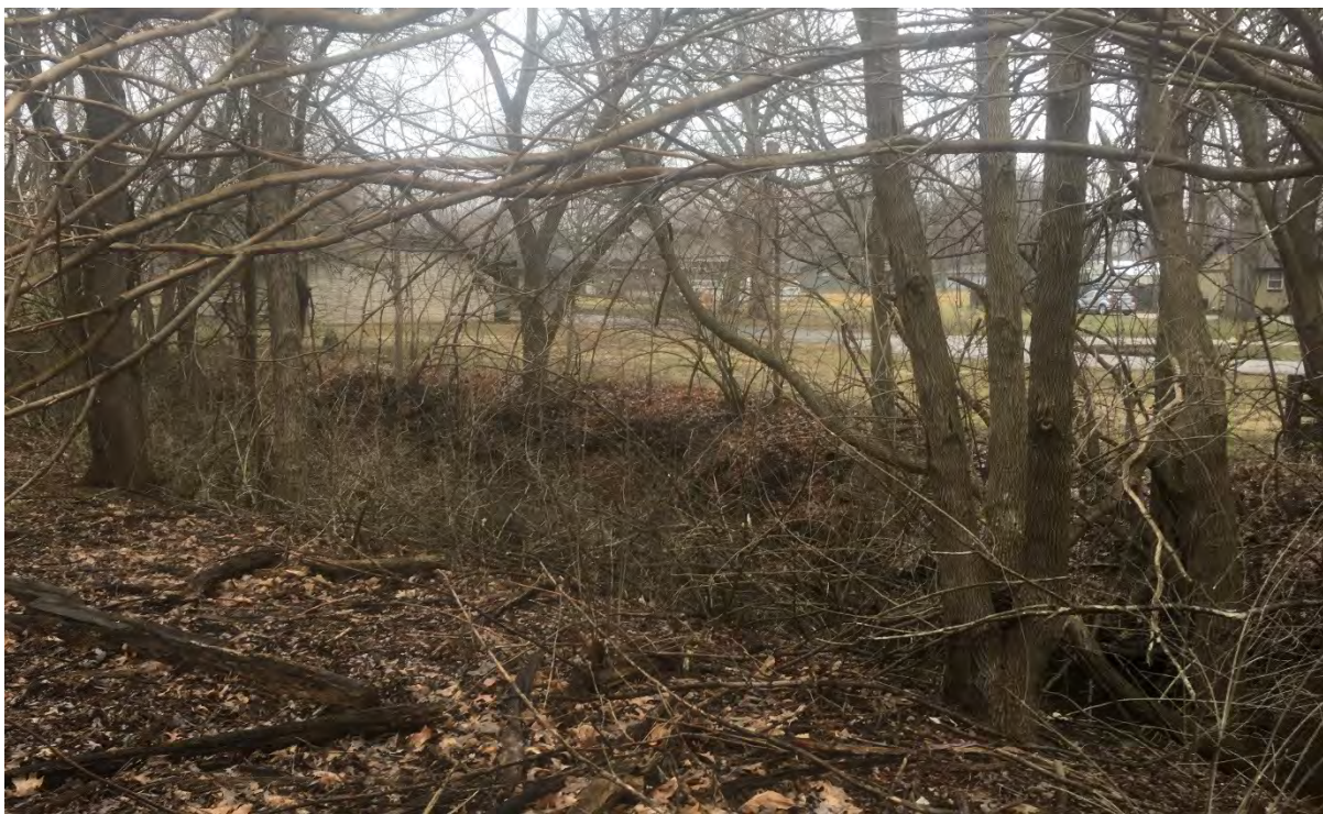
Photo 12: Levee/Elliott Ditch bank conditions, facing west (Location 5)*
