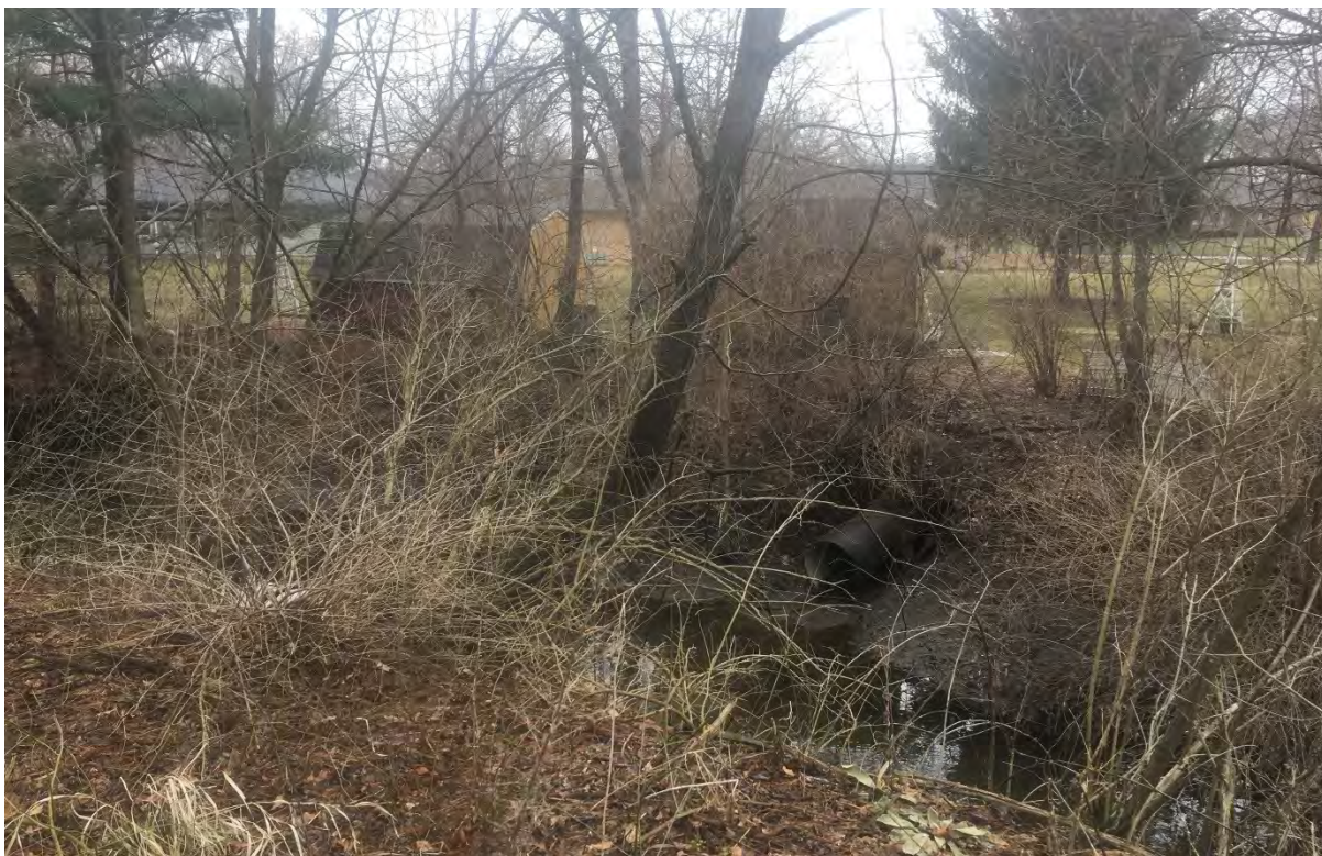
Photo 17: Elliott Ditch bank conditions, facing west (Location 7)*
