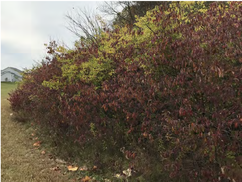
Photo 39: Elliott Ditch bank conditions, facing west (Location 17) (Photo Date: 10/28/20)
