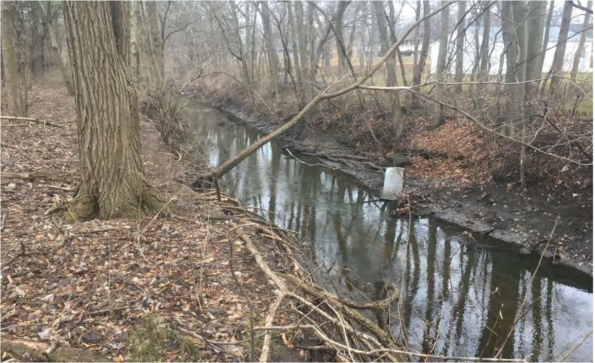
Photo 2: Elliott Ditch bank conditions, facing southwest (Location 1) (Photo Date: 3/21/19)
