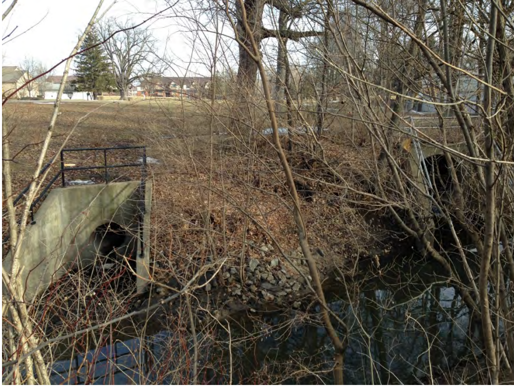
Photo 1: Two outfall culverts on RDB. These outfalls are located on transect 1 at Outfall 001.
