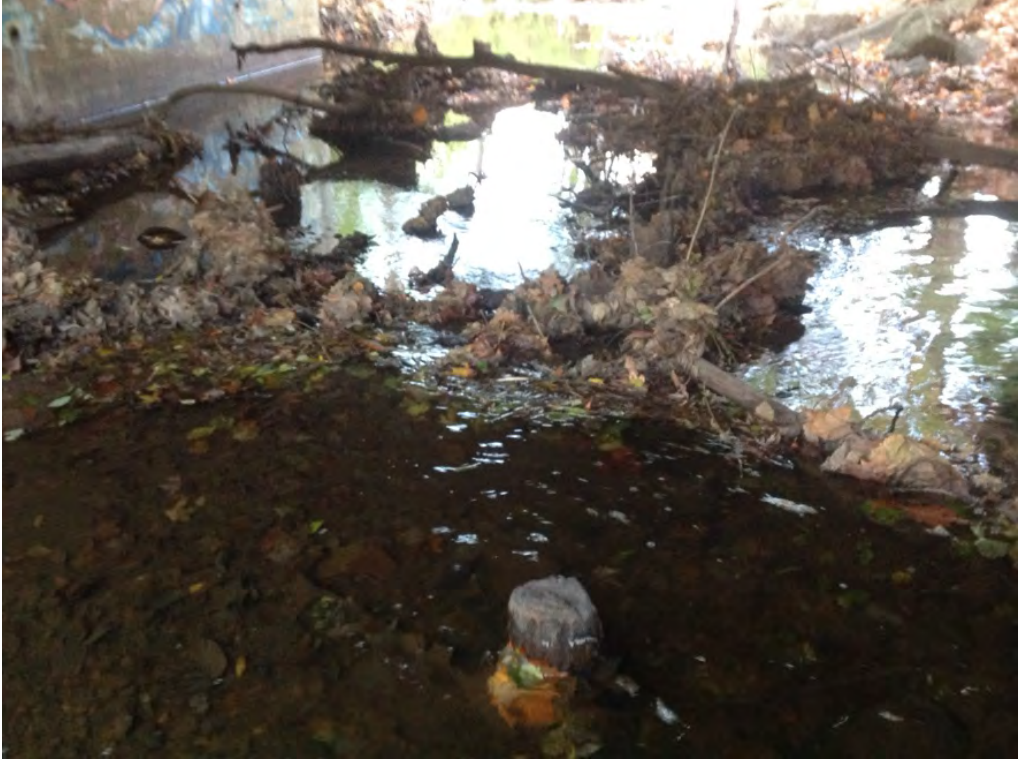
Photo 11: Old wooden bridge pylons and debris under the 9 th Street Bridge.
