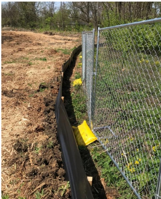
Photograph 1: Erosion Control (Silt Fence) and Temporary Security Fence
